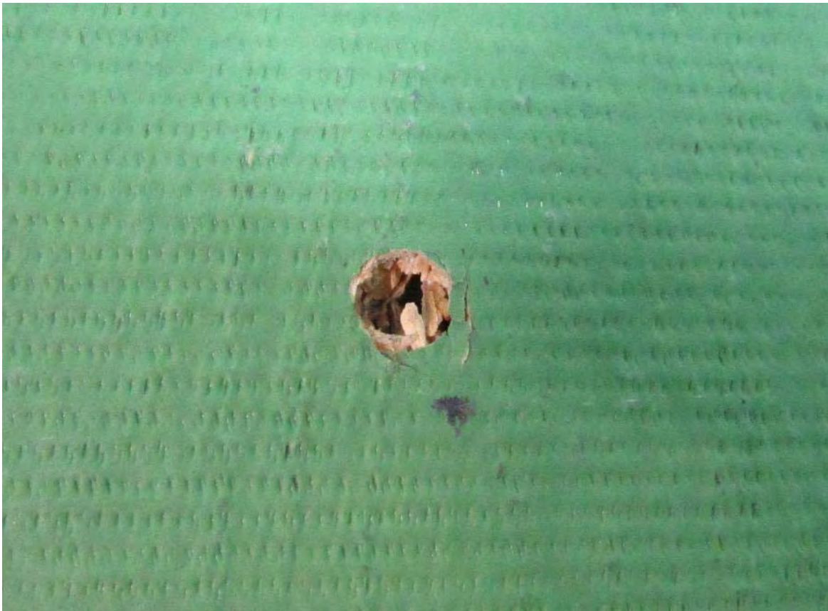
Sample 1 Failure (Sheathing Pull-over Pin Head)
